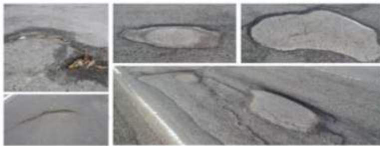
Figure 1: Distresses associated to insufficient bonding encountered on a pavement.
