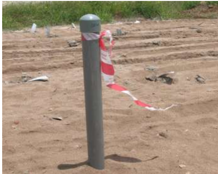
Figure 5 : A Typical Instrumentation protective casing installed on the Embankment.
